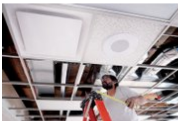
Photo by Hans Hallgren Juan Elizalde, of Air Comfort, installs heating, ventilation and air conditioning into the ceiling Wednesday in the cafeteria at
