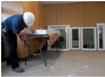
Photo by Hans Hallgren Trenia Reece, of Black Mountain Glass, preps windows Wednesday to be installed at East Elementary School.
